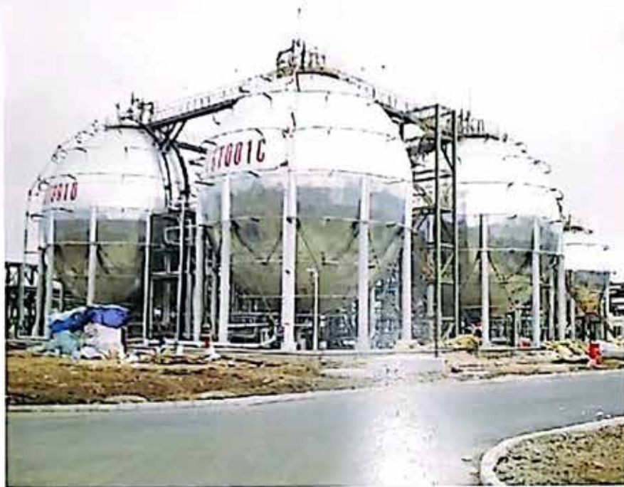
SHEN CHEMICAL INDUSTRY CO. LTD. 2,000 M 3 × 4 SPHERICAL PROPANE TANKS
